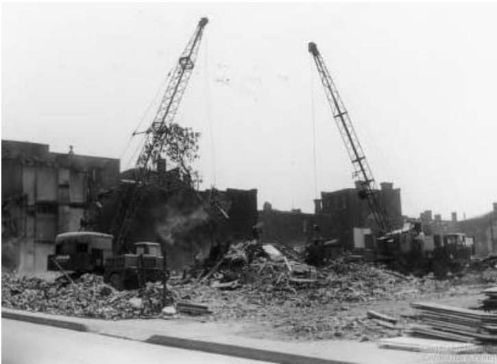
Lower Hill District Demolition. May 9, 1957. Source: Allegheny Conference on Community Development Photographs, 1892-1981, MSP 285, Library and Archives Division, Senator John Heinz History Center
