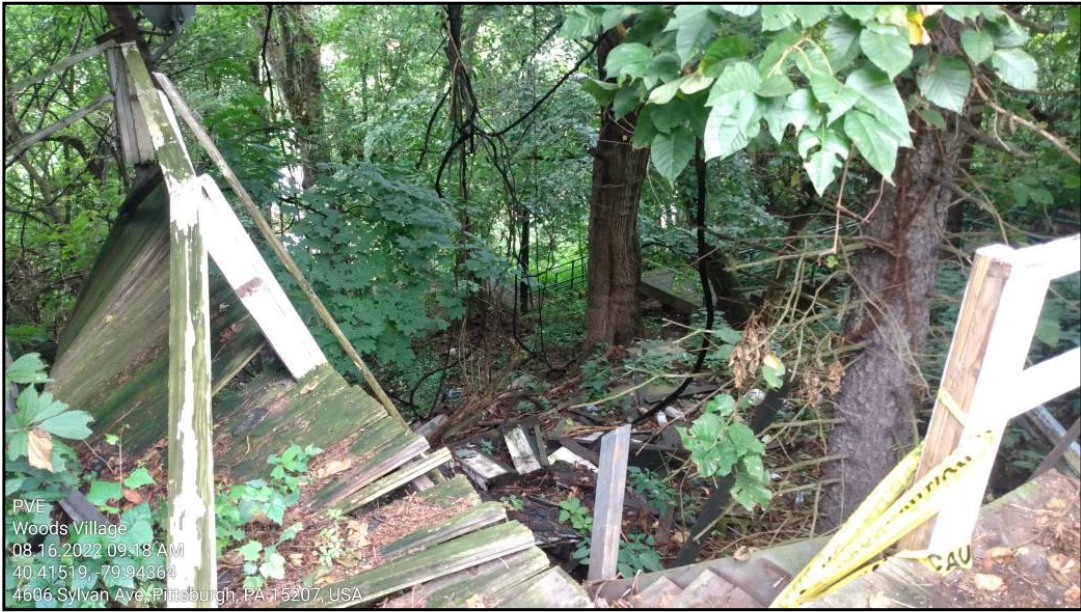
Stairway connected to abandoned structure
