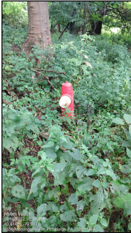
Fire hydrant on Chance Way extension
