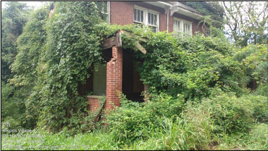
4662/4664 Sylvan Ave. Abandoned structure
