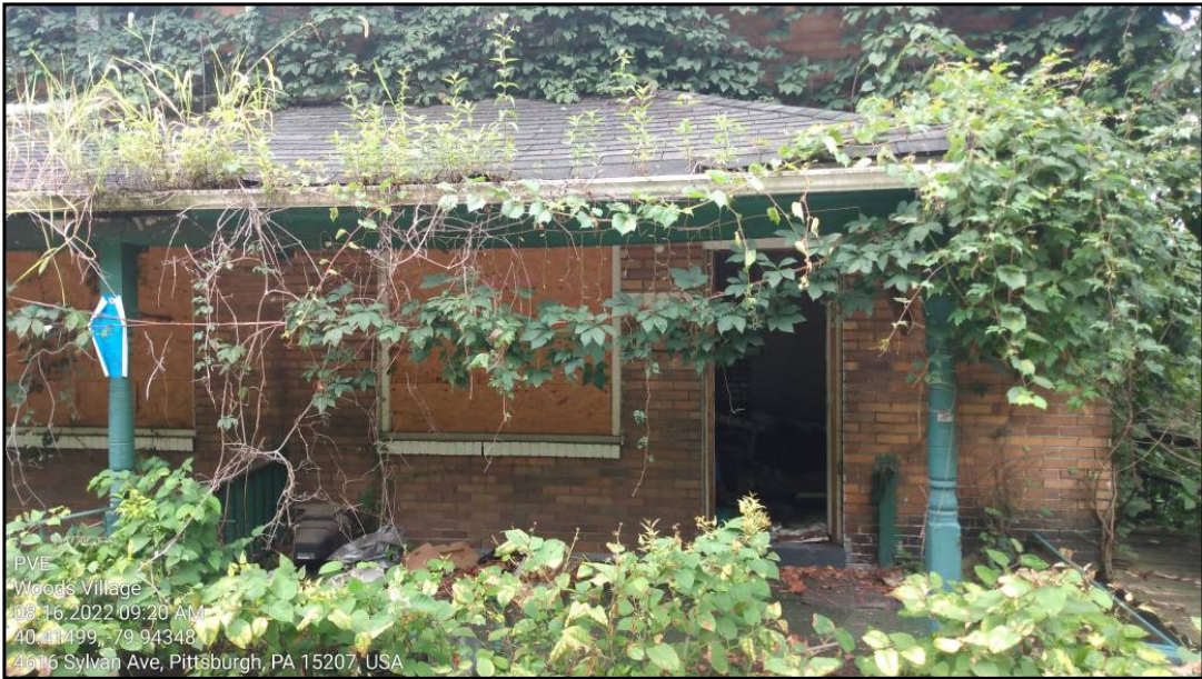
Abandoned structure on adjacent property (4618)
