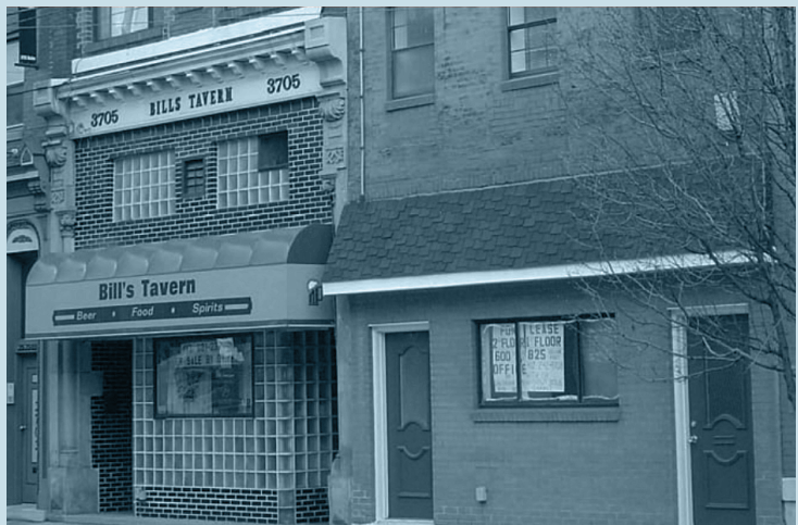
Figure 04. Inappropriate remodeling: closing up storefronts and windows, covering transom windows
